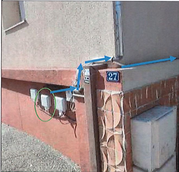
Situation point technique DEPLACEMENT DE LA BOITE
